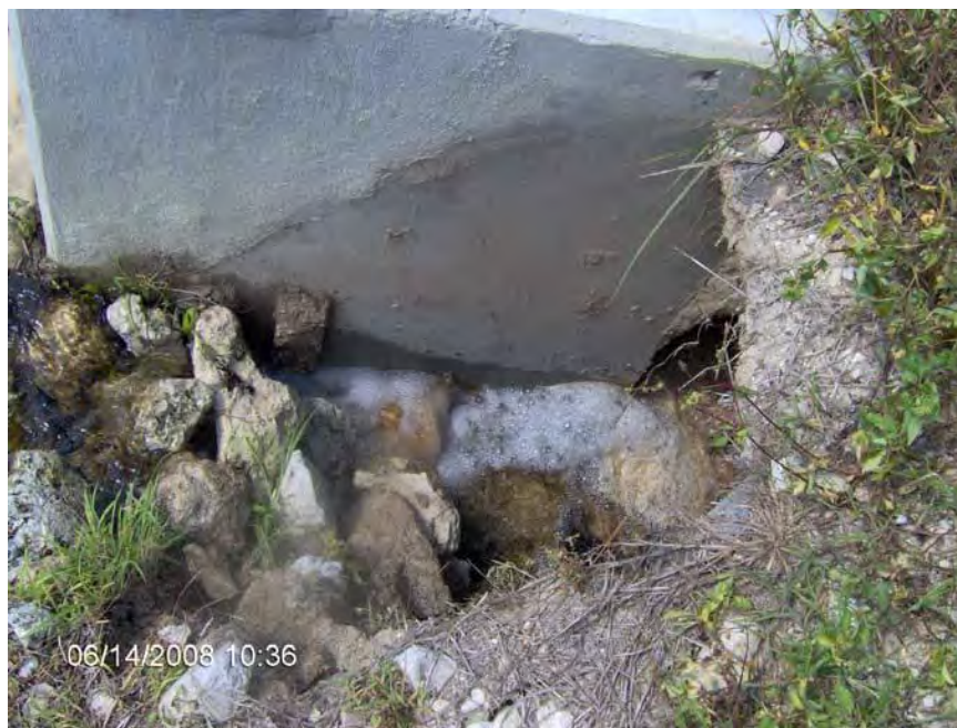
Figure 74: Erosion around the southernmost weir at San Carlos Estates. Source 2008: Exceptional Engineering, Inc.
