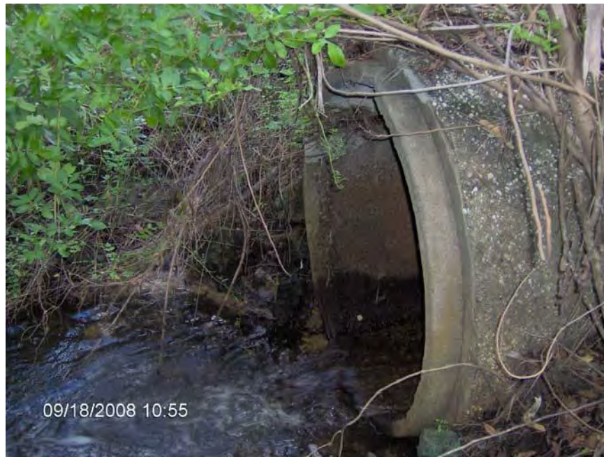
Pic 23. 48" RCP at FPL easement
